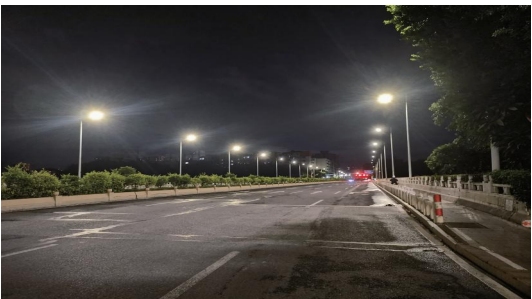
Smart Street lighting project Location:Foshan | Quantity:31,000+
