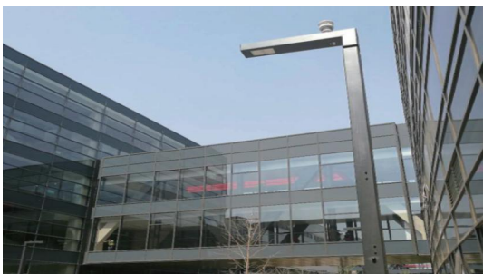
Smart pole project Location: Beijing
