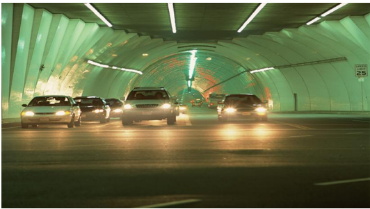
Smart tunnel lighting project Location: Yan'an tunnel in Shanghai
