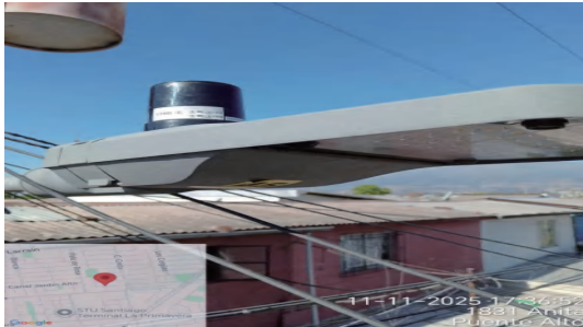
Smart Street lighting project Location:Santiago, Chile | Quantity:40,000+
