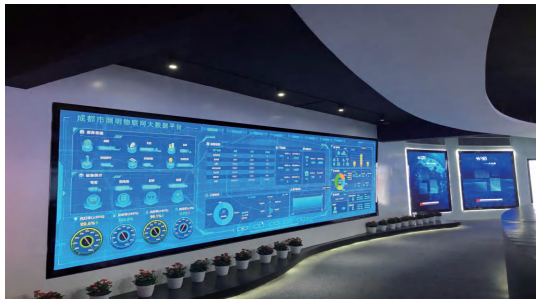
Smart Street lighting project Location:Chengdu | Quantity:210,000+
